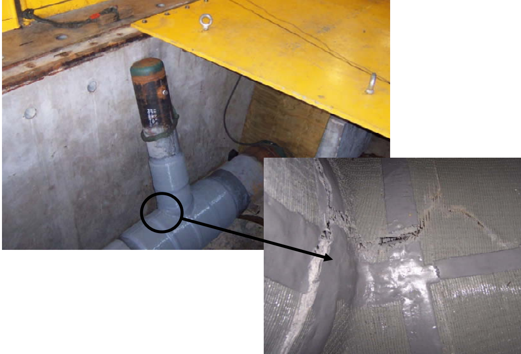
Figure 16 – Leak that developed in composite-reinforced branch connection
